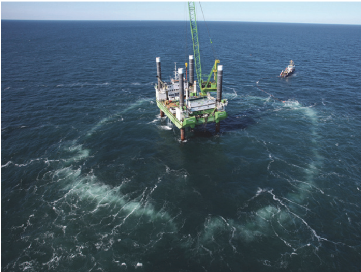
Figure 1. Jack-up installation vessel at OWF Borkum West II surrounded by a BBC from HTL. © Hydrotechnik Lübeck GmbH, source: http://www.hydrotechnik-luebeck.de/bildarchiv/
