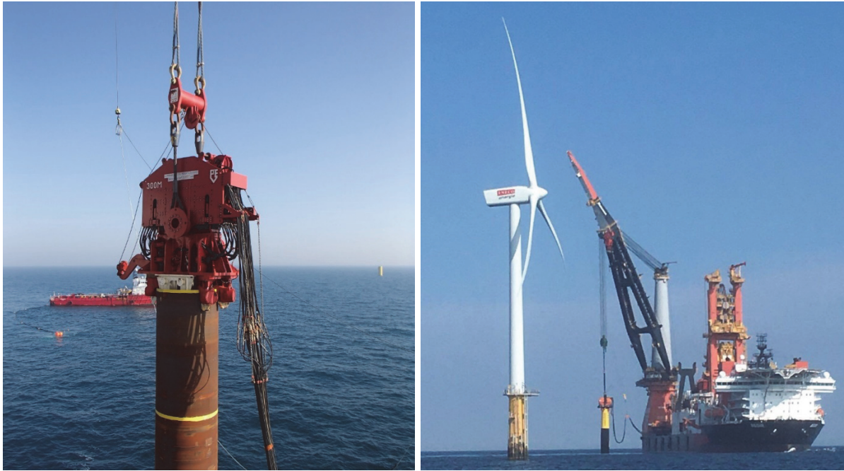
Figure 6. A VH from PVE on a 2.5 m diameter pile used to install a tripod at the OWF Global Tech 1, Germany © PVE (left) and a VH from CAPE Holland vibrating a 4 m diameter monopile at OWF Princess Amalia, the Netherlands © CAPE Holland (right).
